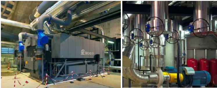
Absorption chiller in the Districlima central production in the Forum area
